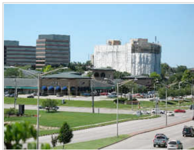
During a recent makeover, plastic covered the Overland Park Marriott, protecting the hotel's customers and their cars from debris.
